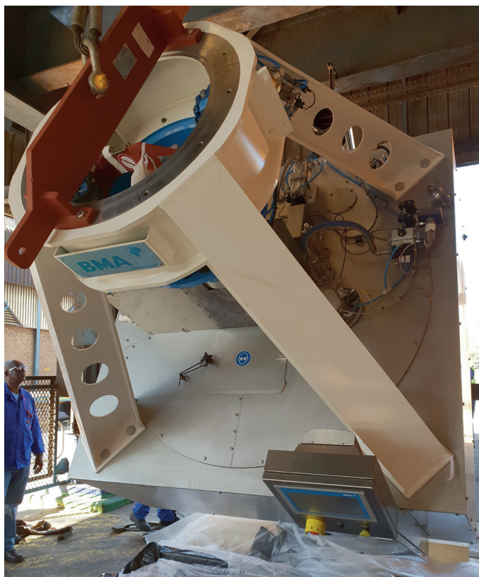
Komati Mill: a new E1810 centrifugal installation
