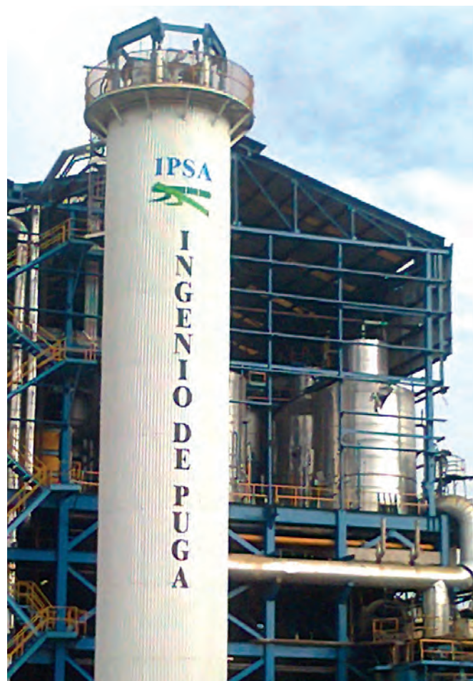
Figure 2. OVC at Puga factory, Mexico
