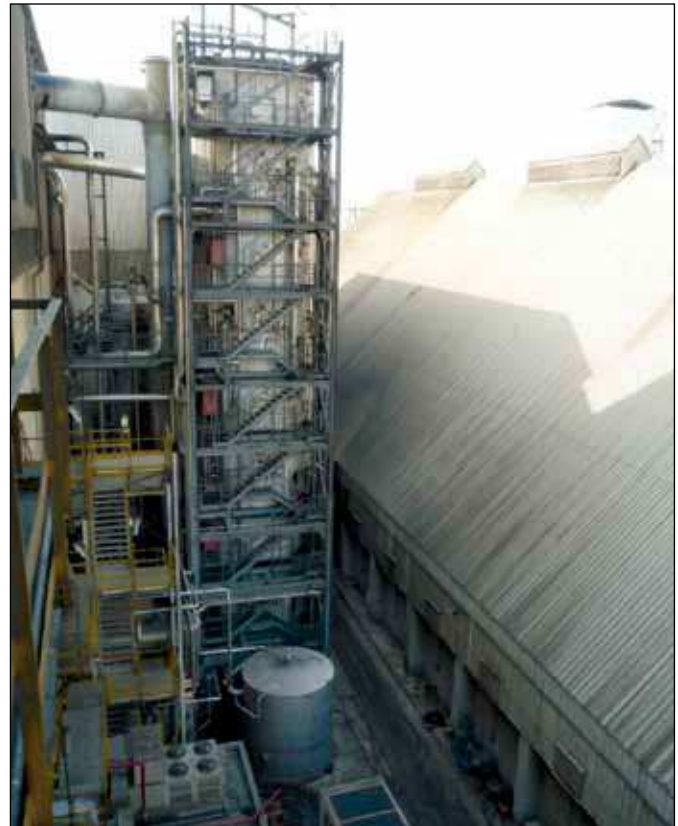
Figure 1. The 31 m tall VKT with the wash water tank in the foreground
